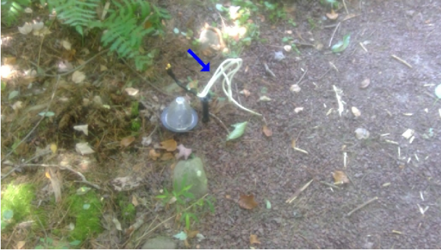
Exposed wiring on walking path to lake also not rated for direct bury
