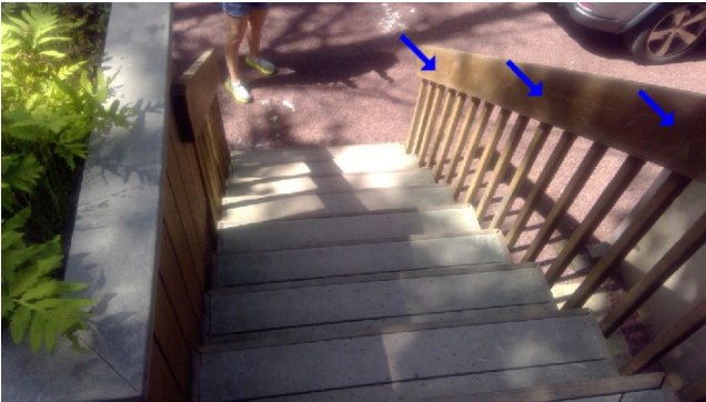
Missing proper graspable rail
