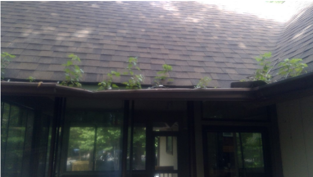
Gutters with debris also damaged
