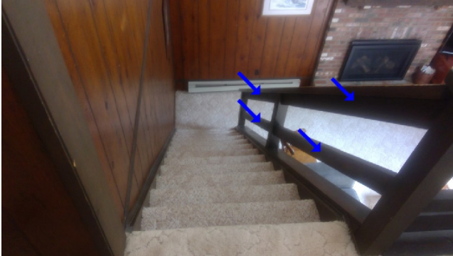
Ladder effect - missing graspable rail
