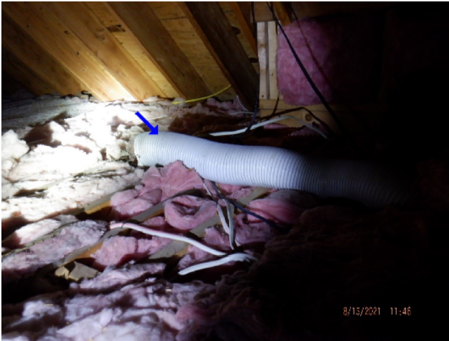
Bathroom fan vents to attic
