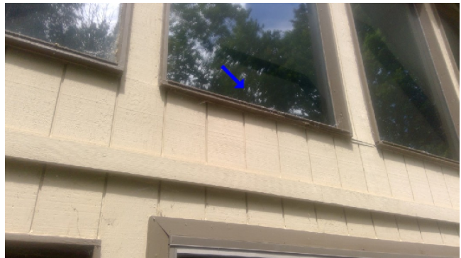
Dry rot at window
