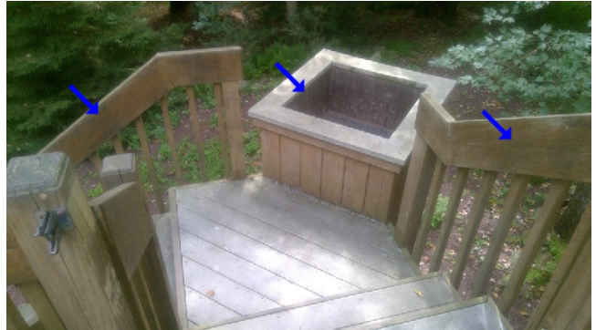
Planter hazard - missing proper graspable handrail
