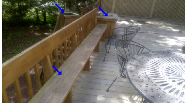
Built in seating hazard / planter safety concern
