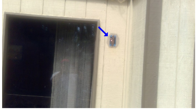
Exposed live electrical wires
