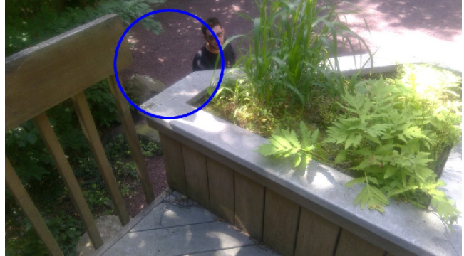
Rails missing / planter box issue
