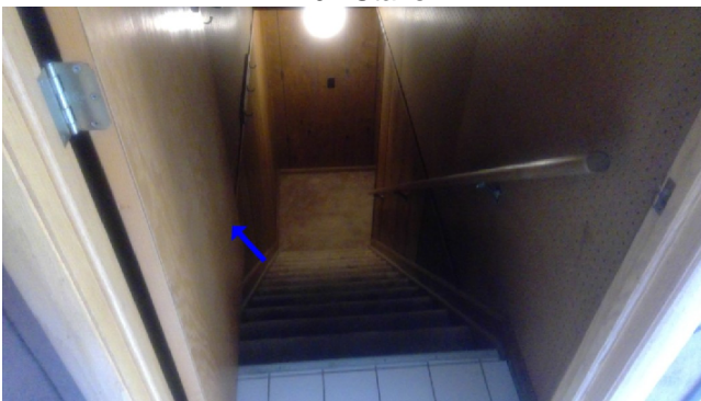
Door swings over the stairwell
