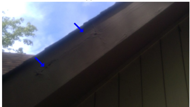
Dry rot at rake trim
