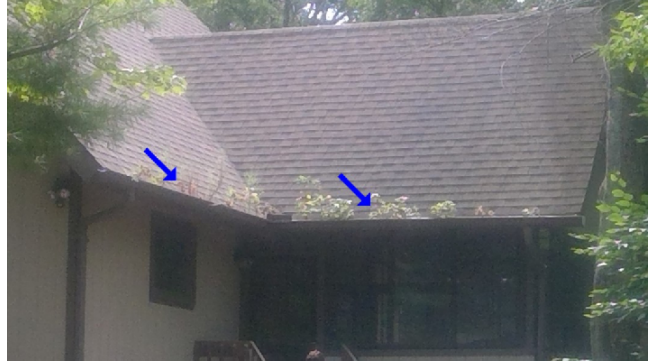
Gutters with debris
