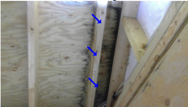
Moisture staining / dry at time of inspection
