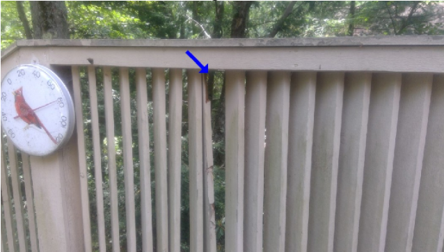
loose board on privacy fence
