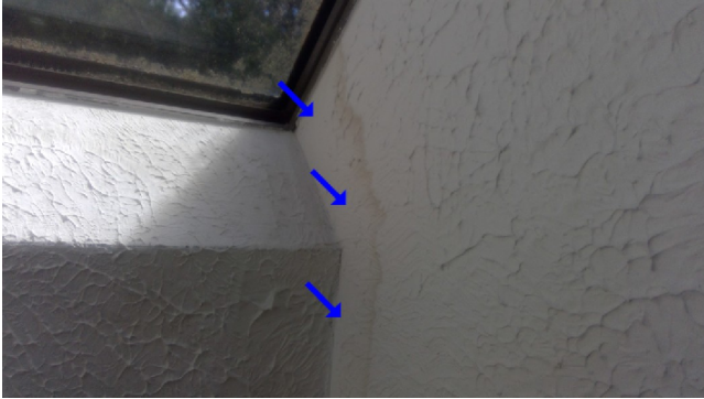
Staining around skylights
