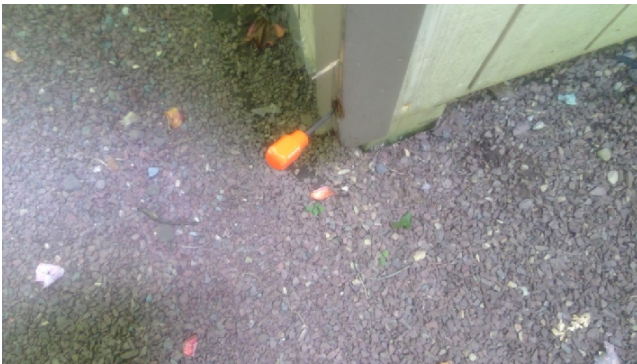
Dry rot by left side shed
