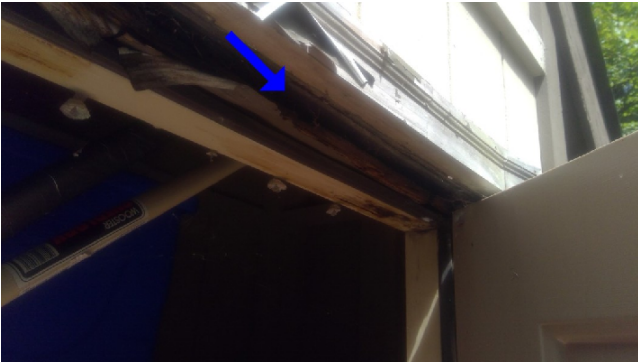
Dry rot around door at deck closet
