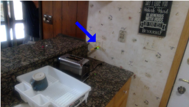
Missing a GFCI outlet
